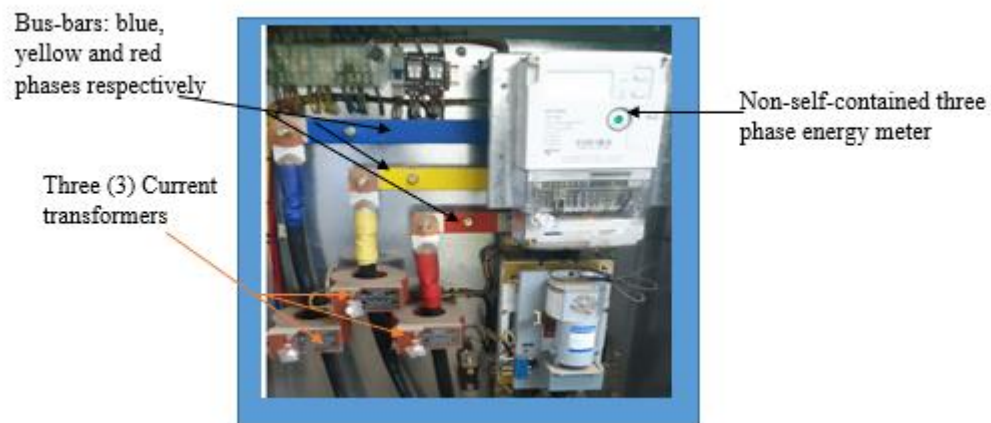
Figure 2: Non-self-contained energy meter and associated three current transformers
